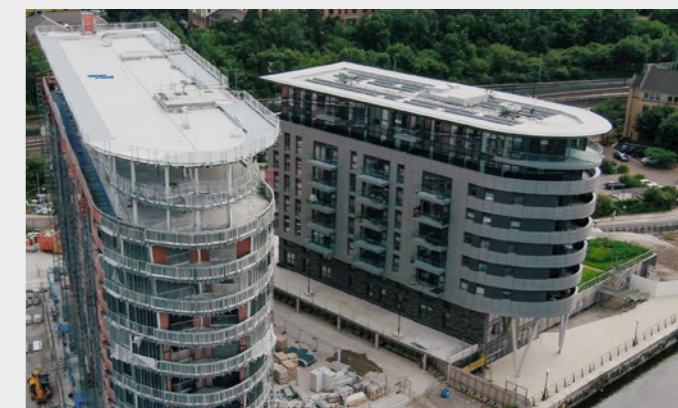
Drone image of the completed Tower A and Tower B which is under construction
